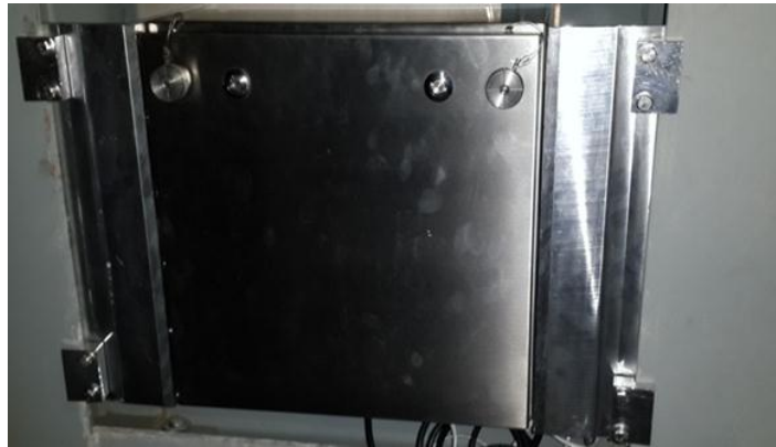
FIG.5. UMS Portal Radiation Monitor installed in the PRIDE facility.
