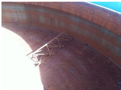
Figure 13 Photograph of the sedimentation tank showing the effect of high iron concentration
