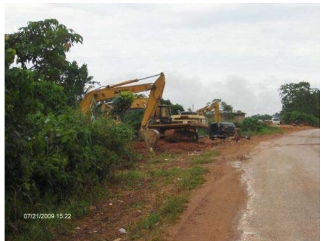
Figure 10. Heavy digging equipment left on the shoulder of the road.
