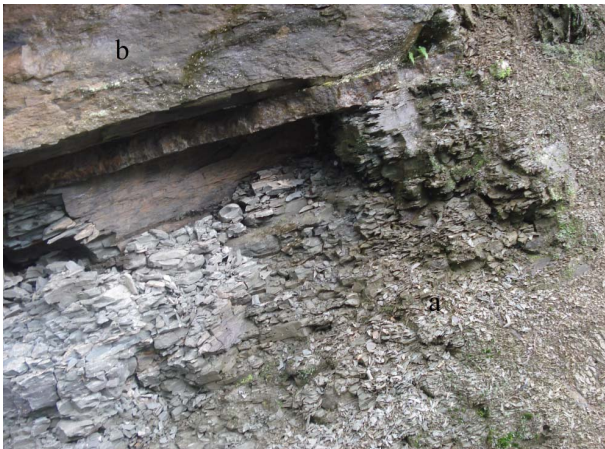
Figure 7. (a) Highly weathered (below) and (b) moderately weathered shale, Yangjia Shan landslide.
