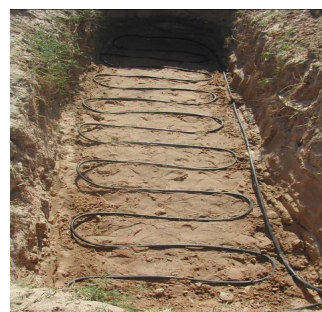
Figure 2. View of the GHE buried at 1 m depth.
