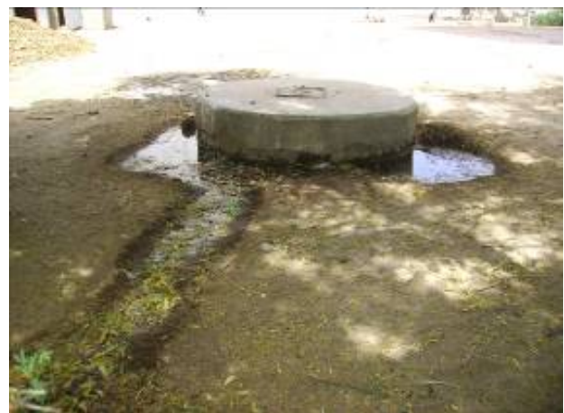
Figure 8. Overflow the pit and creating puddles.
