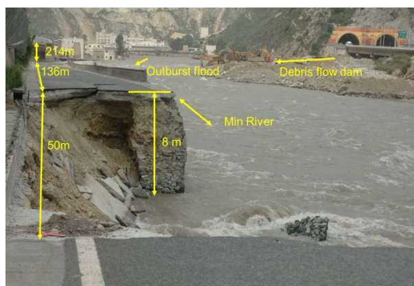
Figure 8. Outburst flood of dammed lake induced by Qipan Gully destroyed Dujiangyan-Wenchuan Highway at the outlet.
