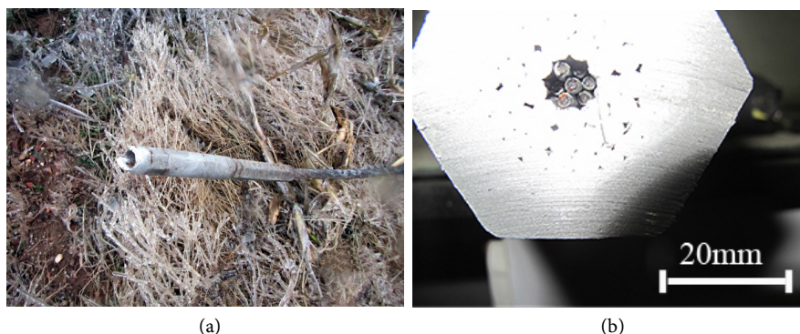
Figure 2. One of the landed strain clamp of 500 kV transmission line (a) fractured strain clamp on site (b) the fracture morphology of the core steels.
