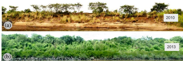
Figure 8. (a) Embankment before implementation of reinforcement works (Sutuli, 2010); and (b) two years after its completion (Hörbinger, 2013).
