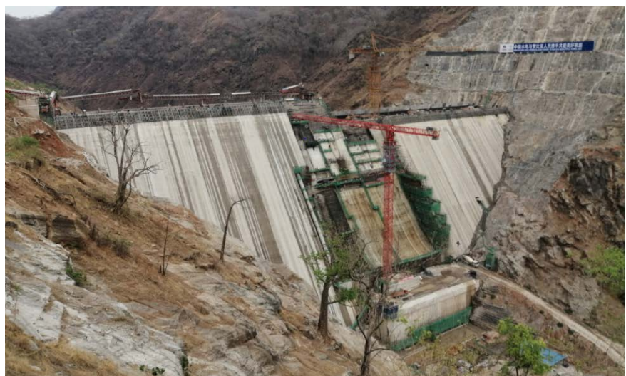
Photo 5. (Downstream) shattered right bank of dam wall.
