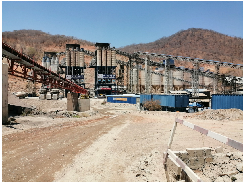
Photo 1. Main crusher and Batching Plants with RCC conveyor Belt (ROTEC).
