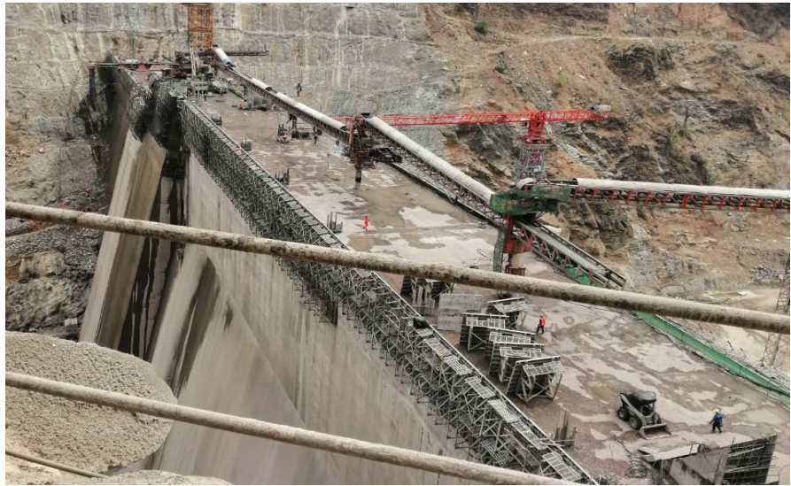
Photo 6. (Upstream) shattered right bank of dam wall.
