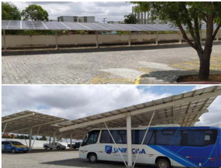
Figure 8. Aerial view of the on-grid photovoltaic solar panel, installed in the parking areas of the University Center of Unifacisa, in Campina Grande, Paraiba, Brazil.
