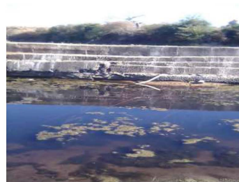
Locally known as ka weir kanini or ka dambwa -made of sand bags or concrete to create an embankment and conserve or harvest rainwater.
