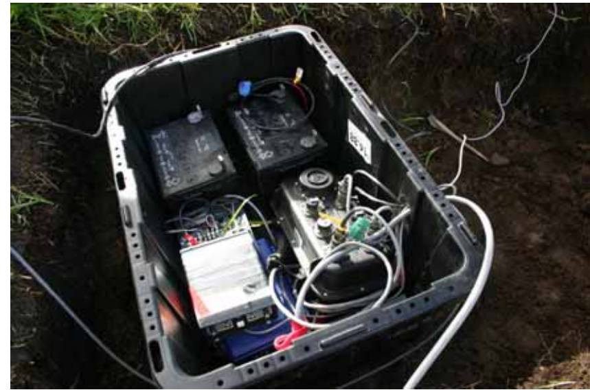
Reventador vent (RVEN) station
