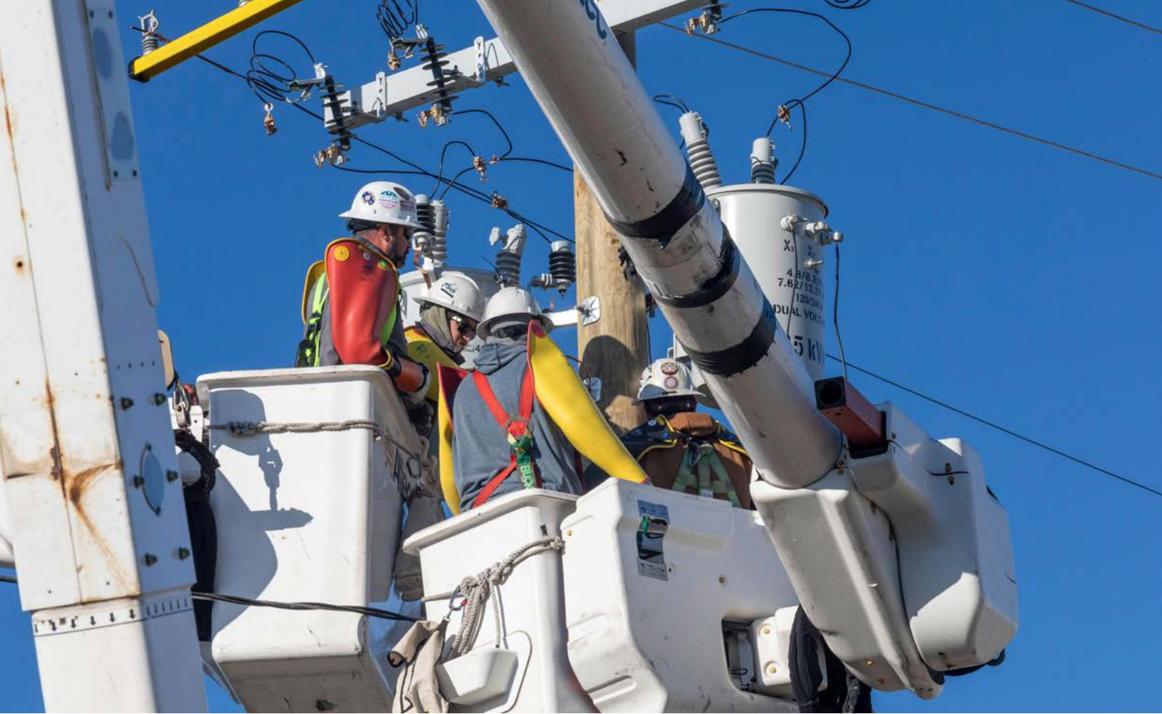
Photo: Electrical linemen, working for DTE Energy, replace transmission equipment on an electrical pole in Detroit, Michigan. Credit: Jim West / Alamy Stock Photo.
