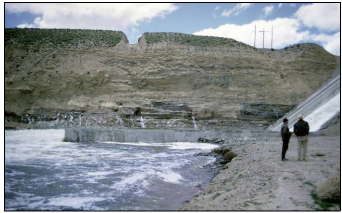
Figure 2B. A photo of the abutment downstream of the spillway. The seepage pattern illustrates the permeability and layering in the foundation.
