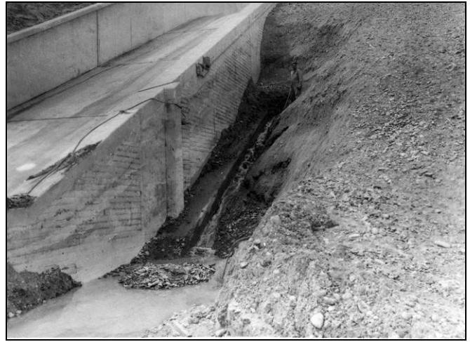
Figure 6B. Seepage emerging from the shale formation along the left side of the spillway chute, May 21, 1965.
