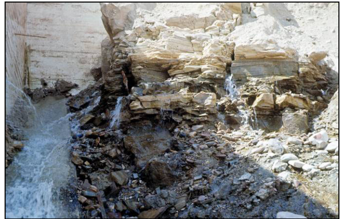
Figure 7B. Seepage emerging from the shale formation along the left side of the spillway chute, July 28, 1965.
