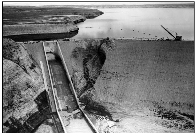
Figure 8B. A wider photo of the large unstable area on the left side of spillway chute, September 17, 1965.
