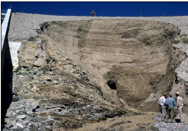
Figure 8A. Muddy seepage emerging from the embankment along the left side of the spillway chute, September 15, 1965.
