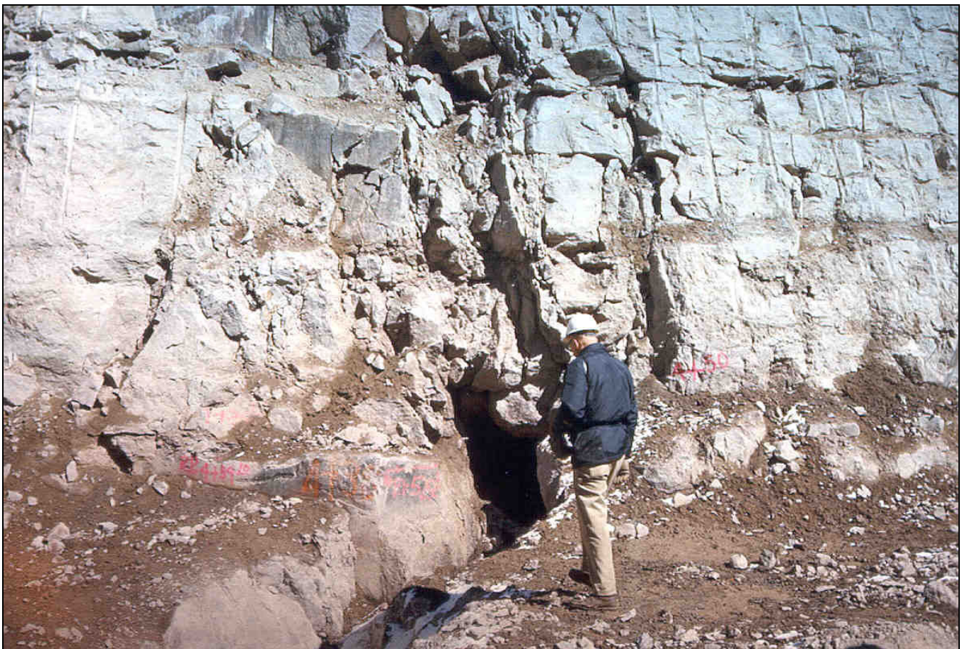
Figure 17. A view of a large fissure in the right abutment key trench
