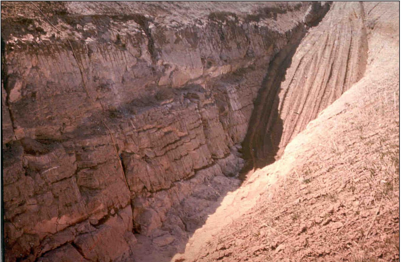
Figure 16. A view of the right abutment key trench showing the jointed nature of the foundation
