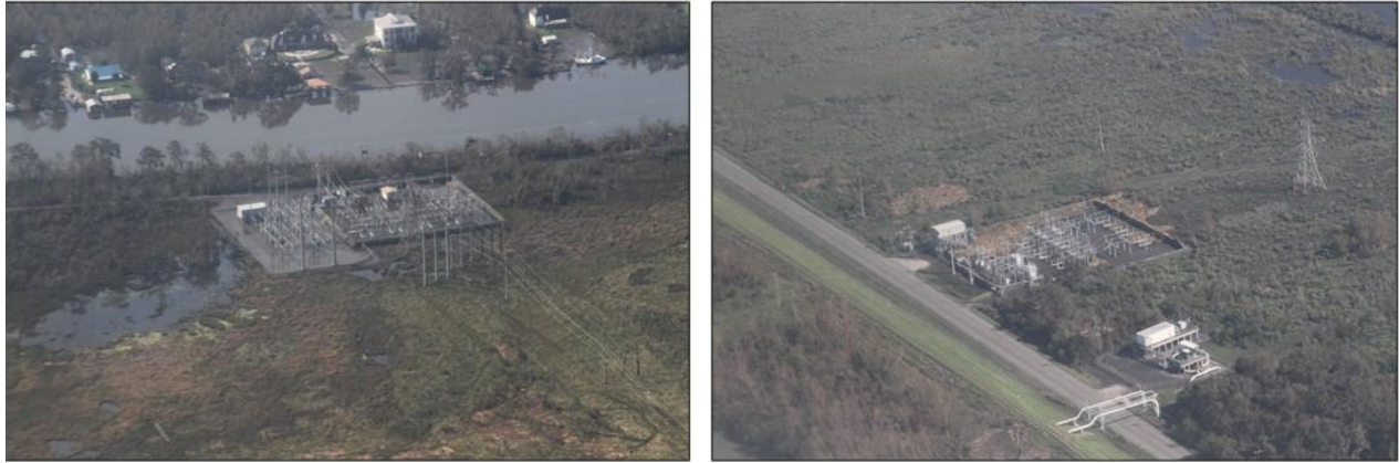
Figure 7. Electrical transfer stations in Plaquemines Parish flooded after Hurricane Ida (04 Sept 2021). Photos: Healthy Gulf % SouthWings.
