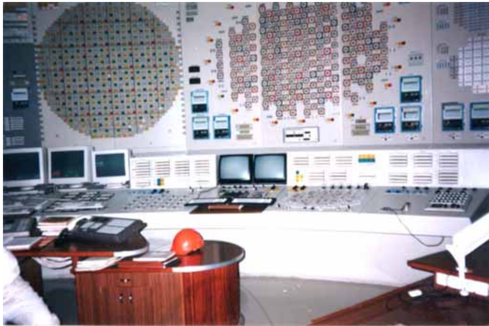
Fig. 2. Control room of NPP unit
