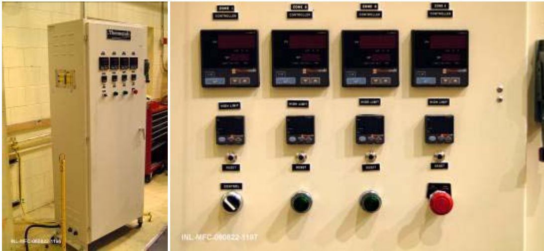
Figure 17. Control Cabinet for Furnace (INL Photo No. MFC-060822-1196 & MFC-060822-1197).
