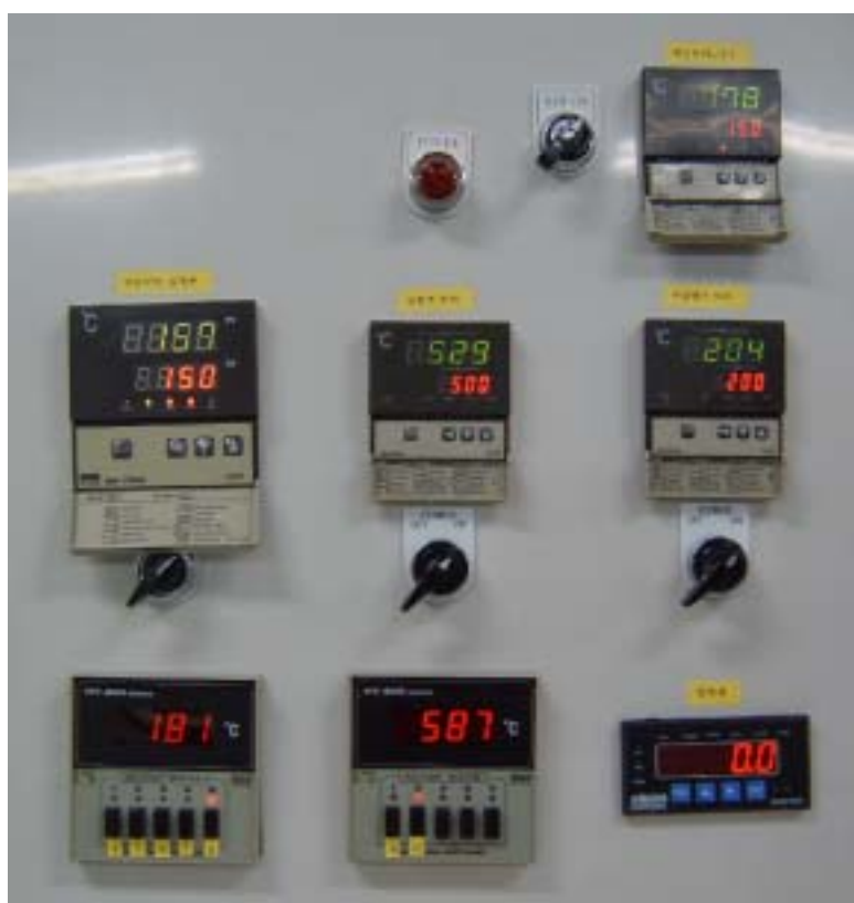
Figure 14. Photo of the control panel.
