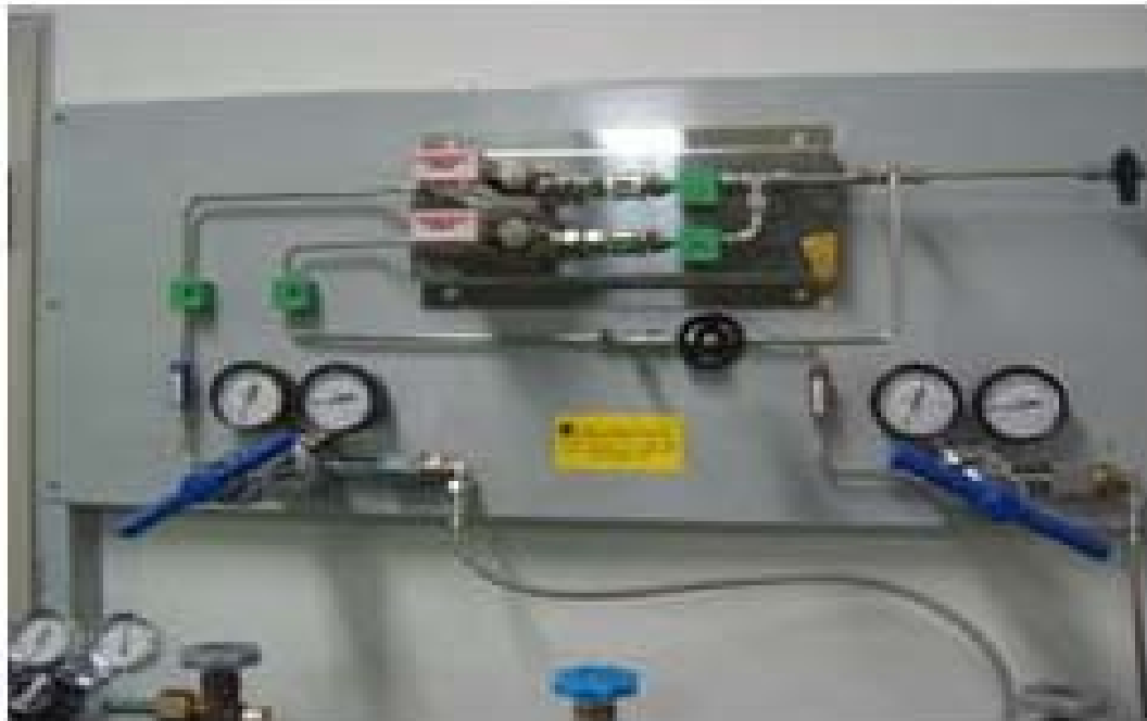
Figure 8. Photo of the mass flow meters (Ar, CO 2 ).
