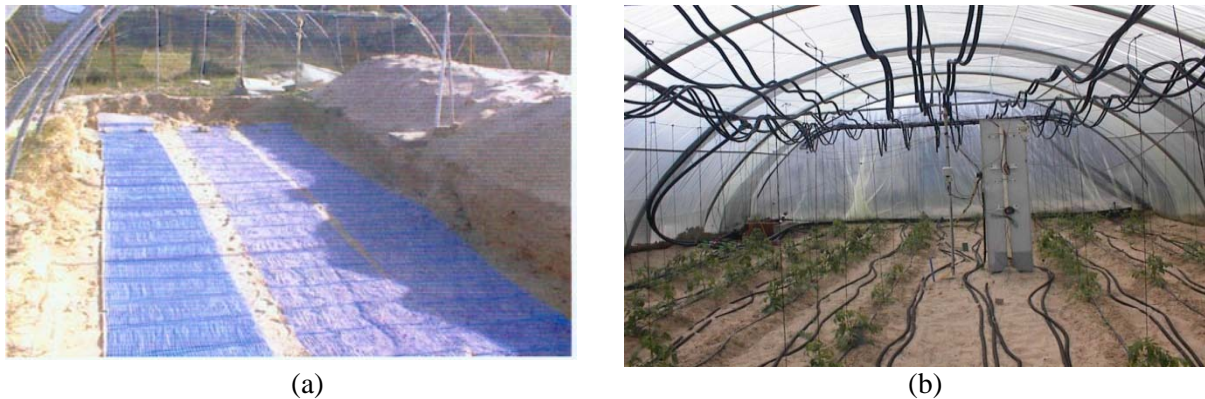
Figure 1. the greenhouse integrated with the designed GHSS: (a) buried capillary plait (b) Agrotherm tubes ringed inside the greenhouse
