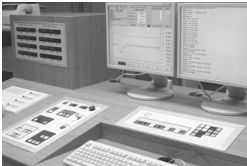
FIG. 2. New operator's desk of the VR-1 reactor.
