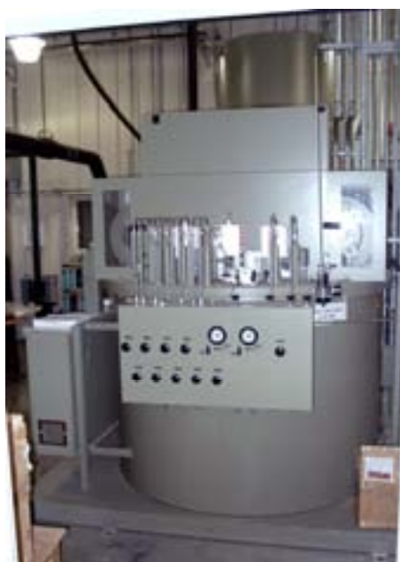
FIG. 14. Helium refrigerator expansion engine pod.
