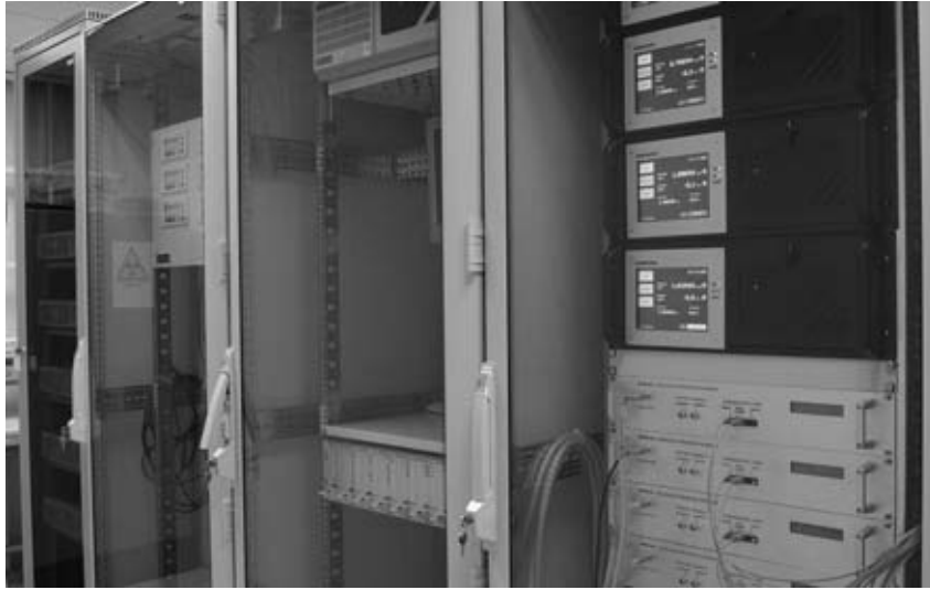
FIG. 3. New I&C room.
