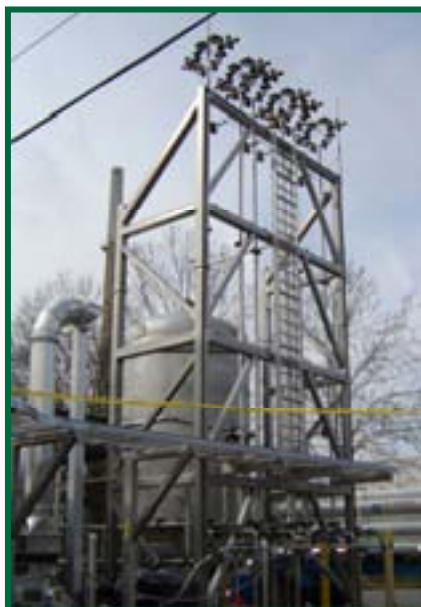
FIG. 16. Relief accumulation vessel and relief stacks.
