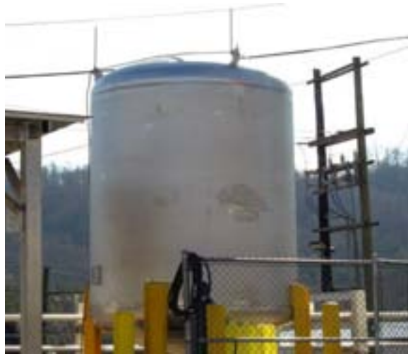
FIG. 10. Hydrogen storage vessel.
