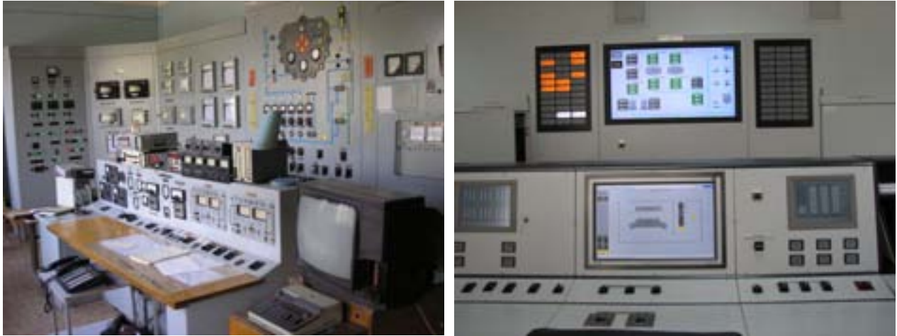
FIG. 3. Reactor control panel: old (left) and new (right).
