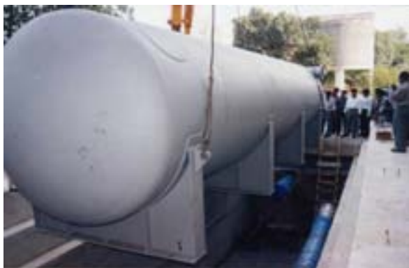
FIG. 3. Installation of the new ^{16}\text{N} decay tank in the decay tank pit.
