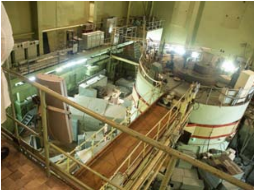
FIG. 1. Common view of WWR-M reactor.
