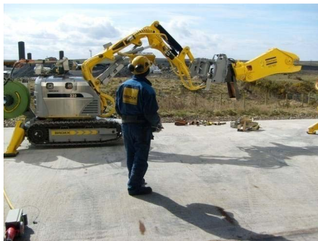
Figure 6: ROV tool commissioning and trials
