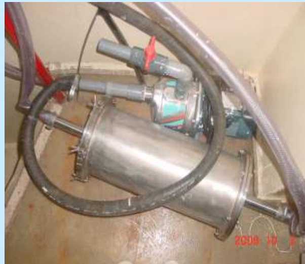
Suction pump of 5 m 3 /h and outside-cover of mechanical filter system
