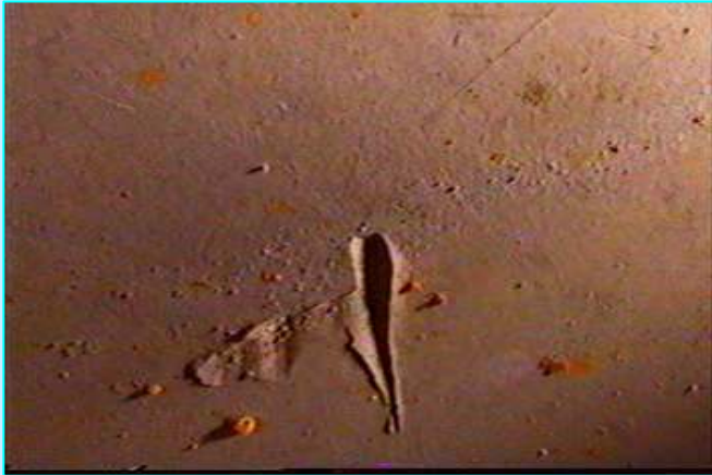
Mechanical defect on bottom of the pool
