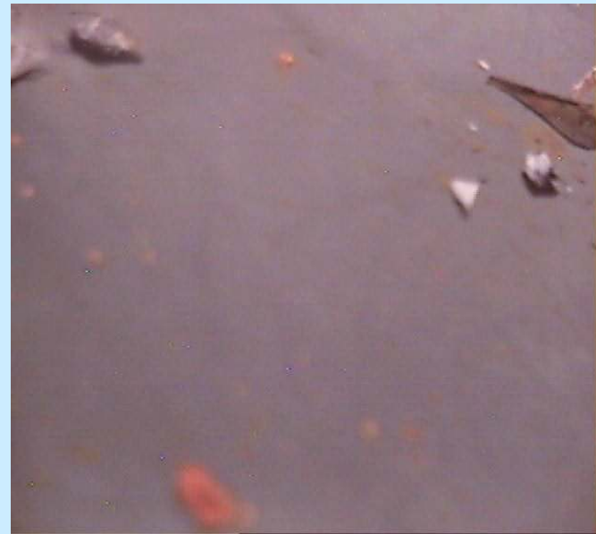
(Some defects on the pool bottom around the reflector leg)
