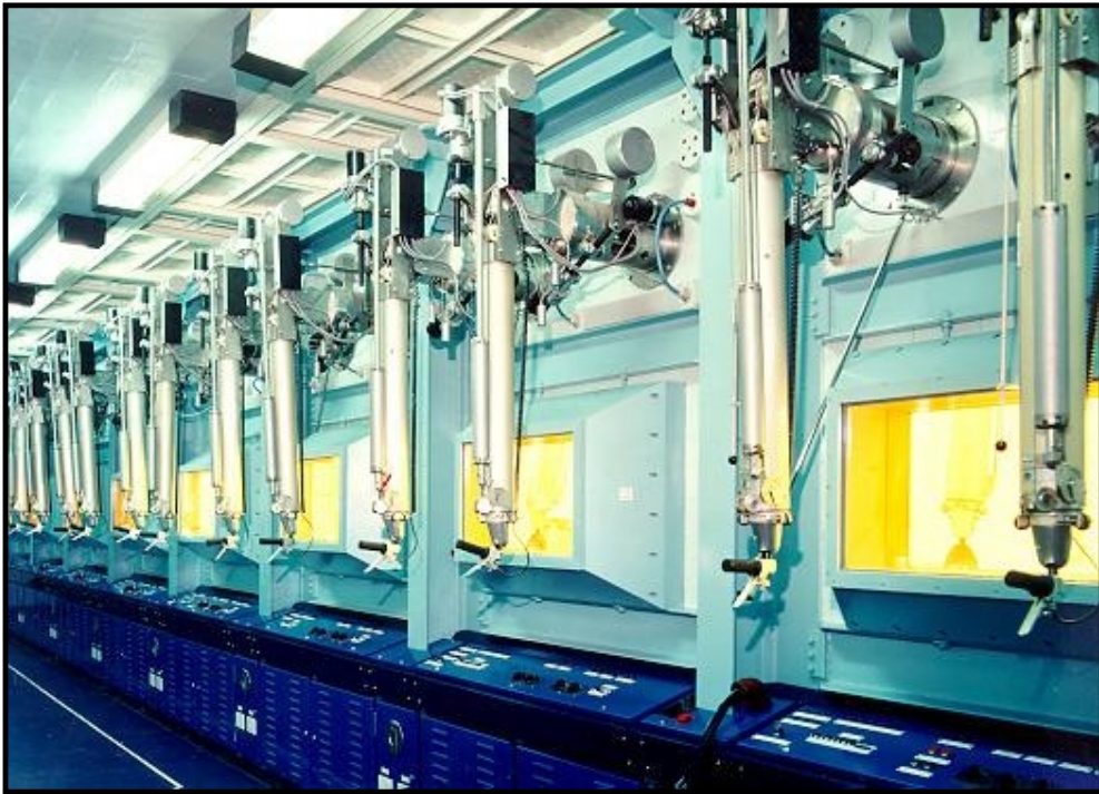
Figure 2: General view of the hot cells at Ezeiza Atomic Center.
