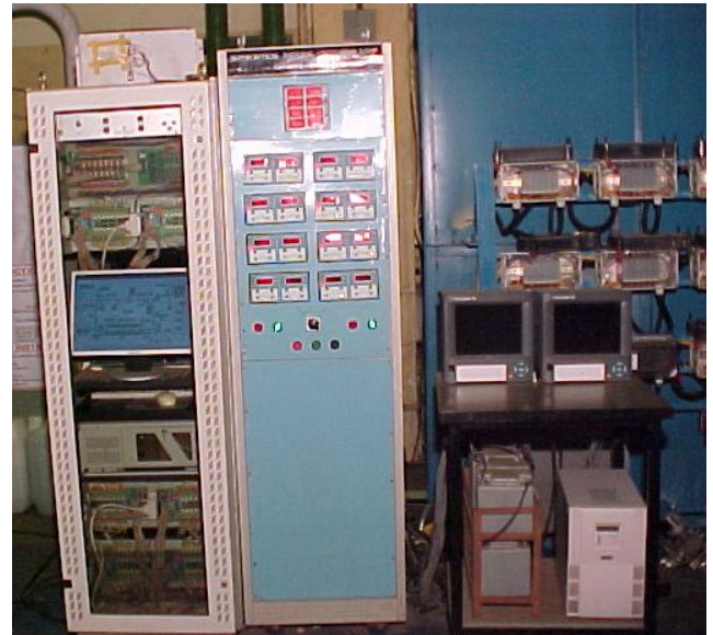
Fig. 4: Photograph of Control Panel for SPNCL
