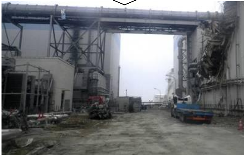
Between Unit 2 and 3
