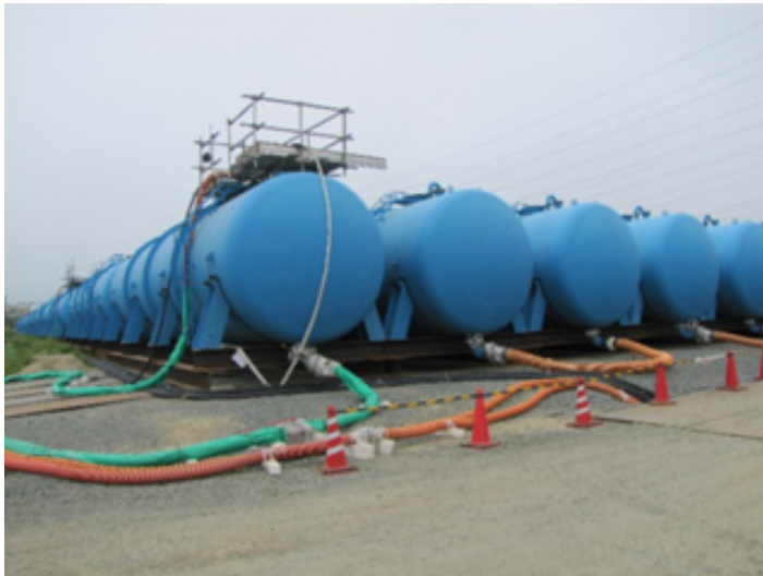
Tank for concentration liquid waste
