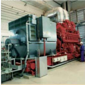
Bar 2, Germany (Konvoi, 1,300 MW) emergency Diesel generator.
