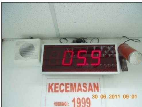
Figure 6: Water level monitor in Control Room
