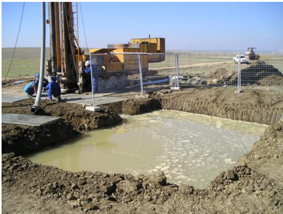
Figure 7. Image of the settling pond used for fluids circulation during drilling.
