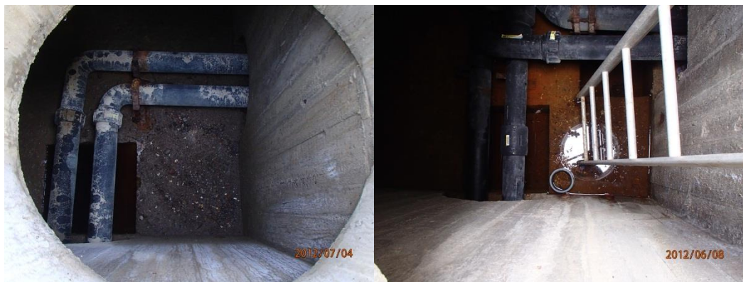
Figure 4. Well shaft in two manholes in non-viable part of the active pipes (with and without ladder).
