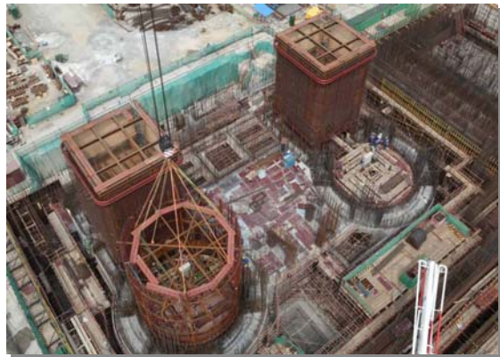
Module B of CWS for reactor cabin
