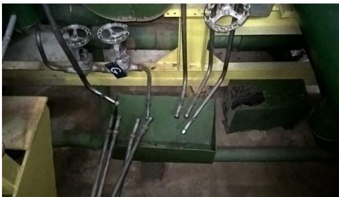
Fig.2. The air discharge and effluents discharge/collecting pipes from testing rigs – partial view
