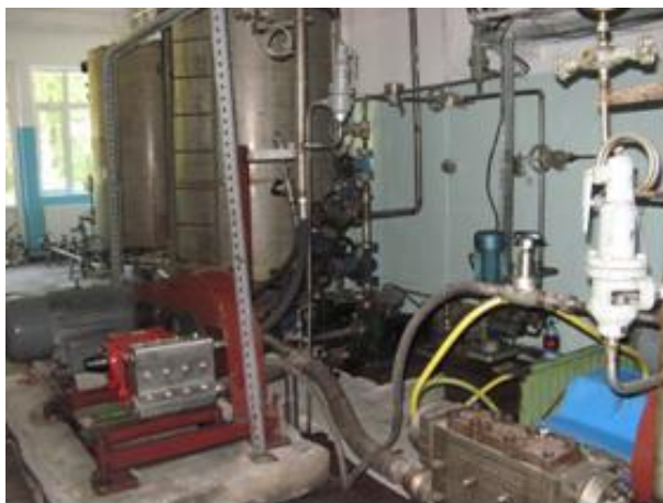
Fig.2. The water treatment station – partial view
