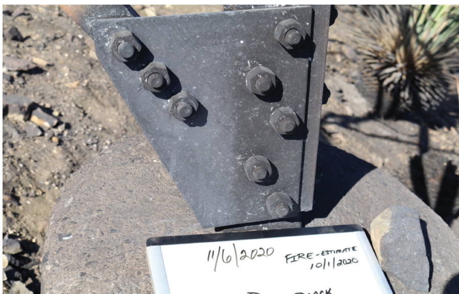
FIGURE 2 A tower leg foundation after exposure to a wildfire. Note spalling of the concrete foundation.
