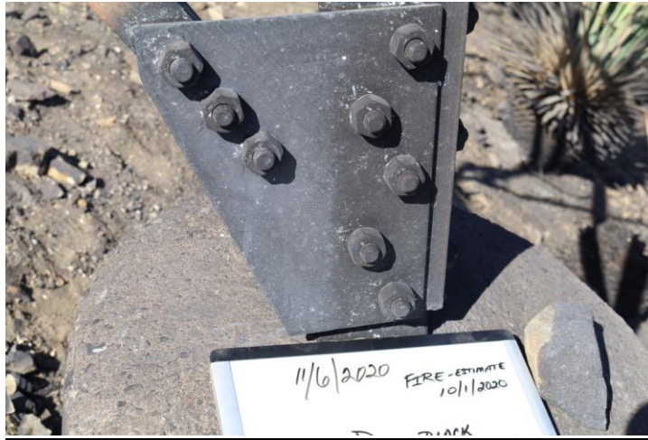
Figure 7: Photograph of a tower leg foundation after exposure to a wildfire. Note spalling of the concrete foundation.
