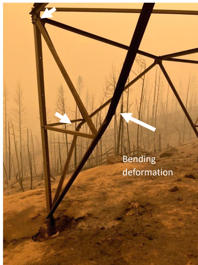
Figure 4: Photograph showing the deformation of two diagonal steel braces and one instance of a bolted joint pulling away from vertical structural member (upper left). The other arrows point to the inflection points of the deformed diagonals.
