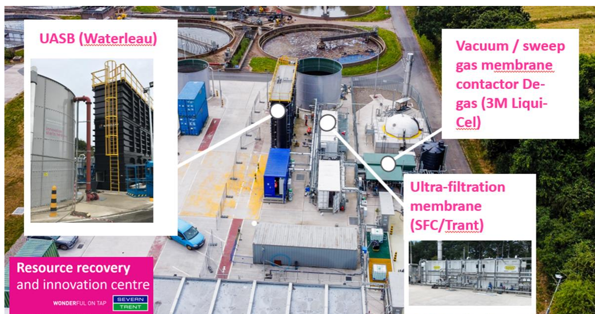
Fig. 2 NextGen: UASB full-scale plant in Spenal with UF and degassing unit
