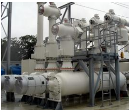
ELK-14, 362 kV 1½-breaker arrangement
