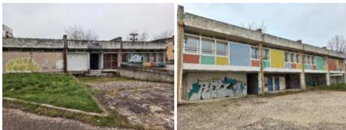
Figure 26 View of a) the North facade (left) and b) the South façade (right) of the building
