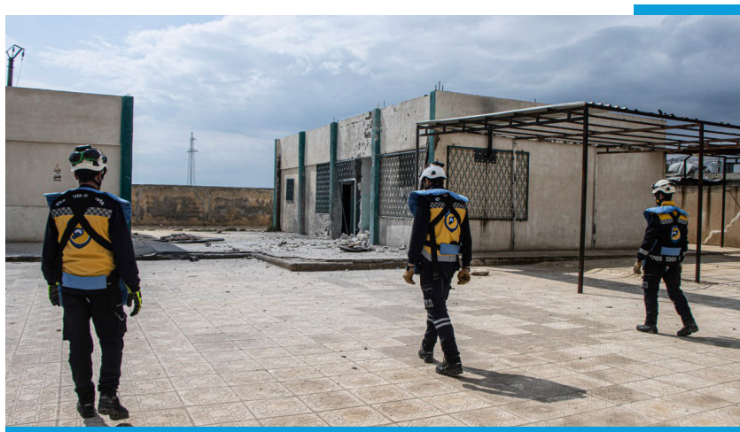
↑ Destruction caused by a ground regime attack Murshed Mohammad Ayyan Elementary School in Katyan village in Idlib - March 19, 2024
