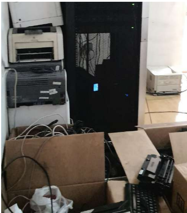
Figure 42. Server Room in Yerevan Erebuni District Court (exemplary)
