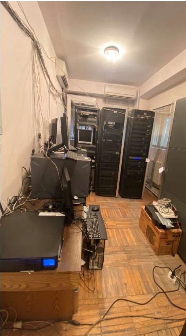
Figure 41. Server Room in the Yerevan Court of Appeal
