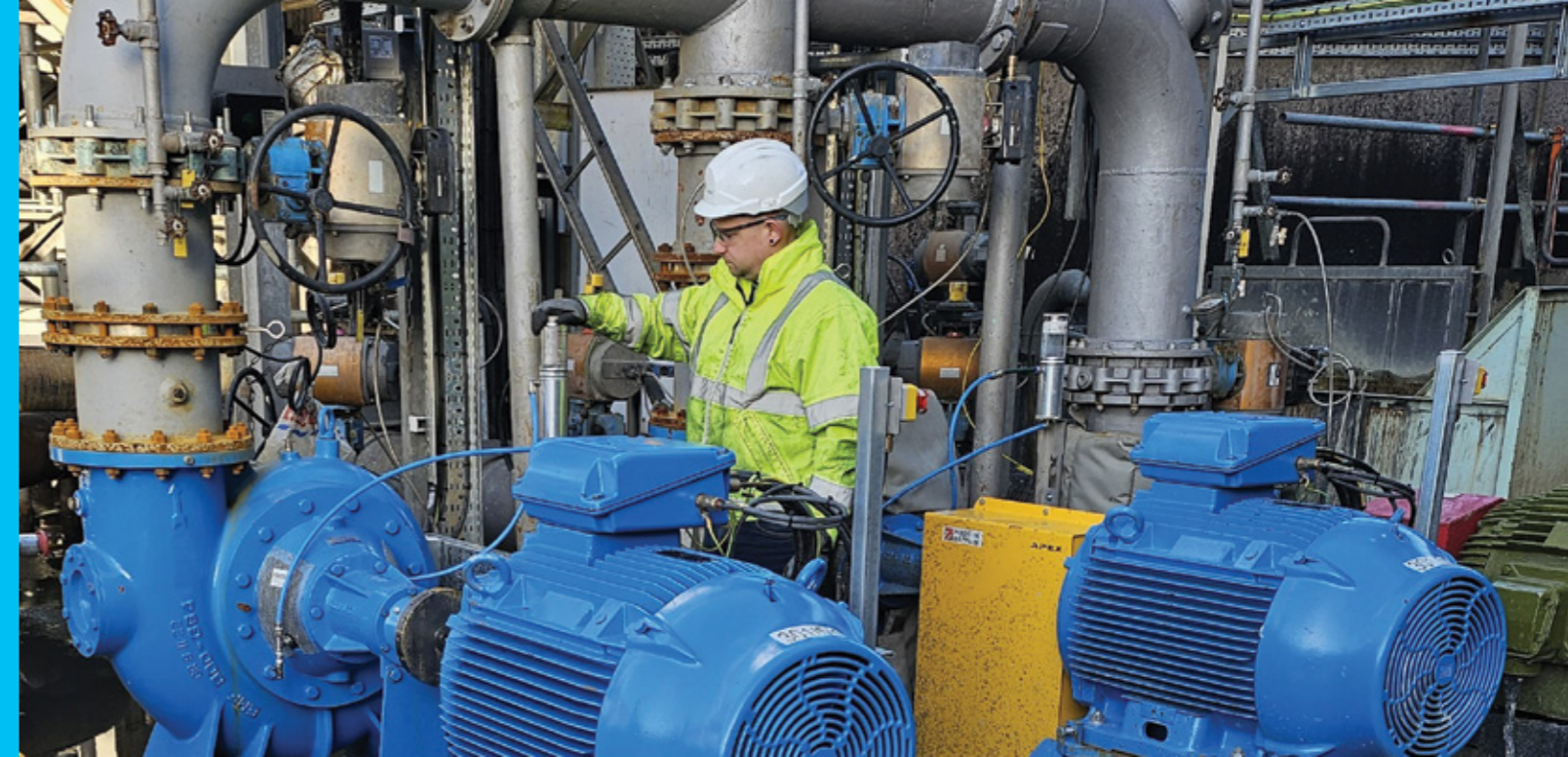
Mark Fish, Senior Coordinator of Production, checks the new VSD pumps in our Effluent Plant.
