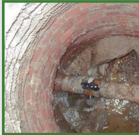
Broken sanitary sewer
