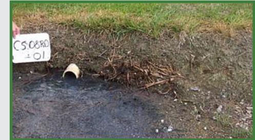
Cheater pipe from septic field
