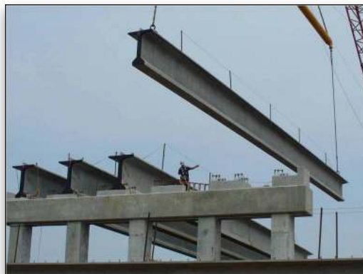
More than 345,000 linear feet of prestressed-precast girders were designed with LEAP CONSPAN.
