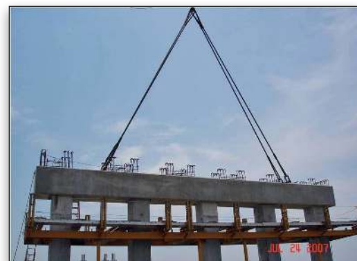
Precast reinforced concrete caps designed with LEAP RC-PIER were used for the majority of the spans.
