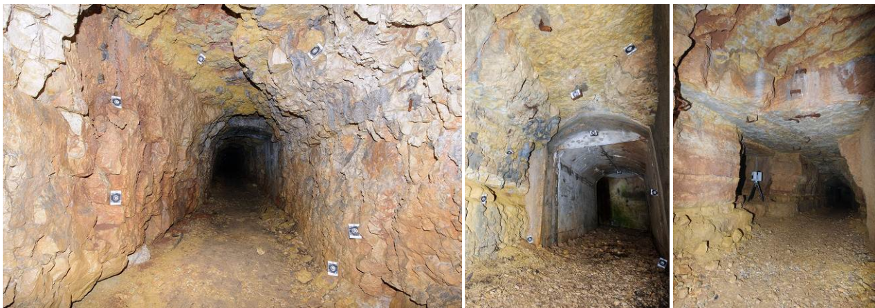
Figure 2. The tunnel - connecting the Viaz and Oberwiesen outposts of the Lusern fortification - with the topographic targets (left and middle) and a TLS station (right).
