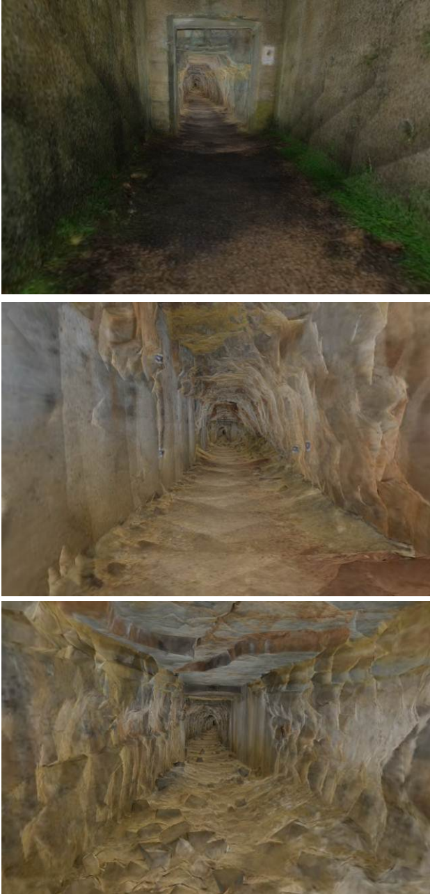
Figure 9. The final photorealistic 3D model of the tunnel, with the texture applied over the sharp optimized 10 cm mesh.
