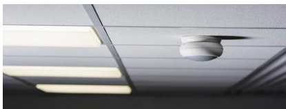
Security, environment control
