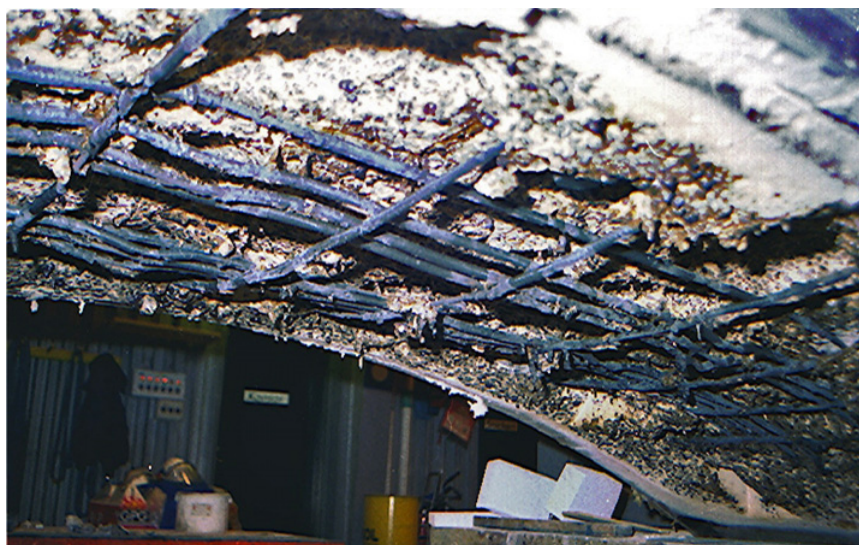
Figure 2. Tunnel element from the Great Bealt tunnel fire tested at SP Technical Research Institute of Sweden. Photo included in the official report from the Danish Transport Authority [39].
