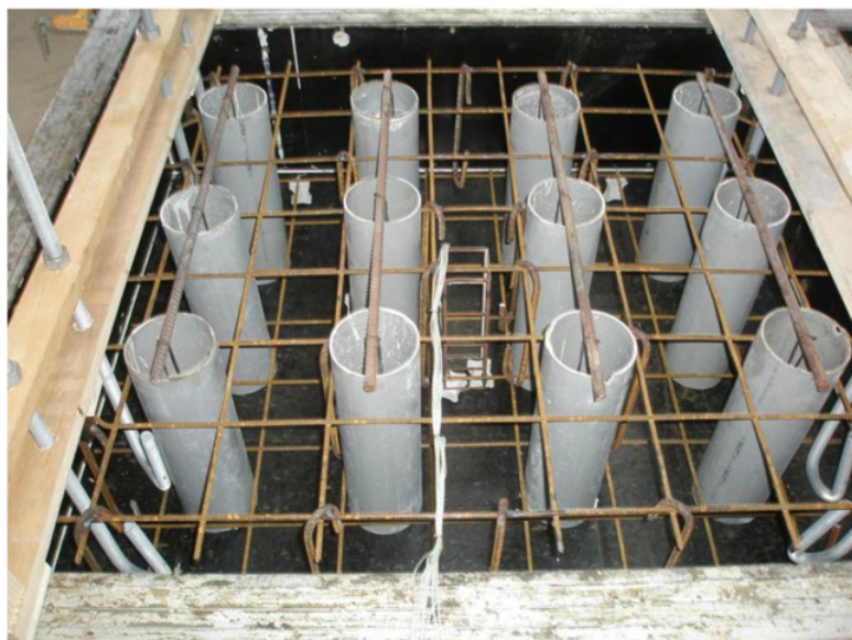
Figure 1. Pictures of the slab in which will be embedded cores, before the casting.
