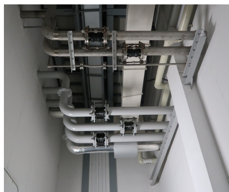
Figure 6: Rubbers for vibration isolation are inserted in the middle of cooling pipe.
