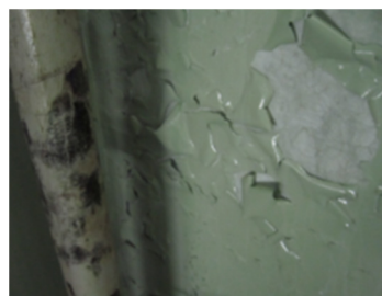
Figure 2: Peeled epoxy coating at \mu -monitor.
