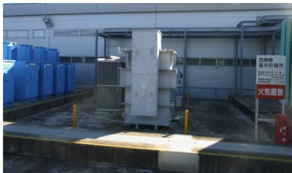
Figure 9: Storage location of the transformer-rectifier unit.
