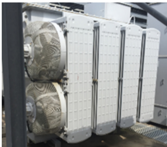
Figure 2: MR-RF transformer-rectifier unit.
