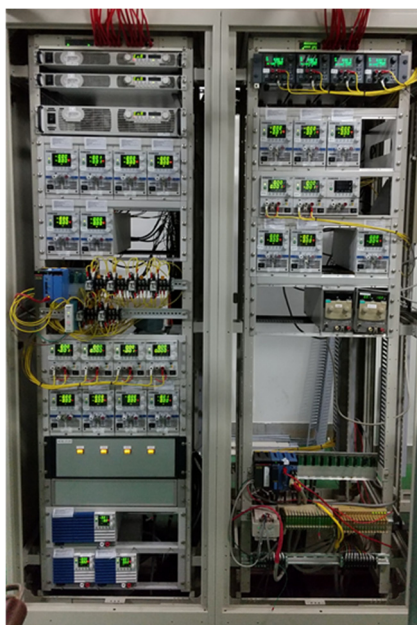
Figure 2: Photograph of new power supplies for magnets.
